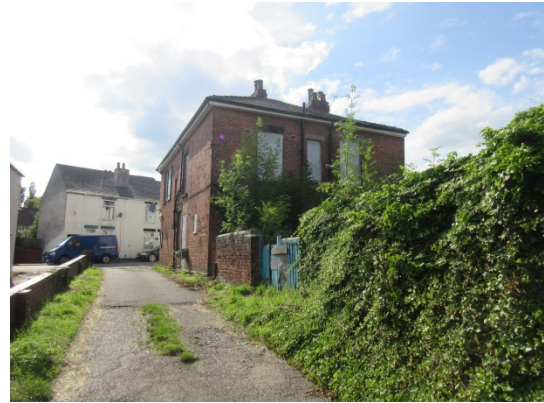
Rear (east) elevation and south (side) elevation of the site, taken from Devonshire Villas
